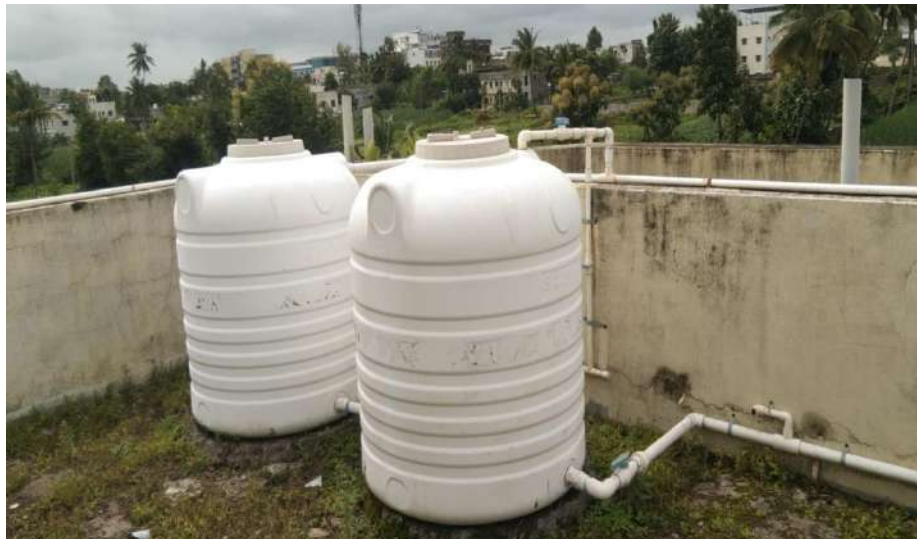
Water Tanks in College Campus
